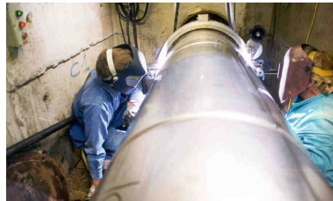
Stainless steel inserts as a repair solution for underground main supply lines. Source: Centro Inox (Italy), www.centroinox.org
